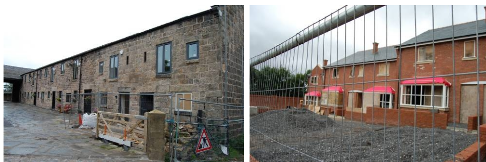
(Left) Conversion underway to Bidston Hall Farm (Right) Construction in progress on Bidston Village Road
