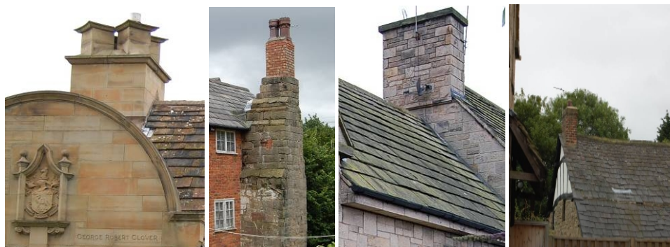
Chimneys in the conservation area; (1) Clover Cottages (2) stone with sections rebuilt in brick seen extensively (3) simple copings to stone chimneys(4) plain brick stack.
