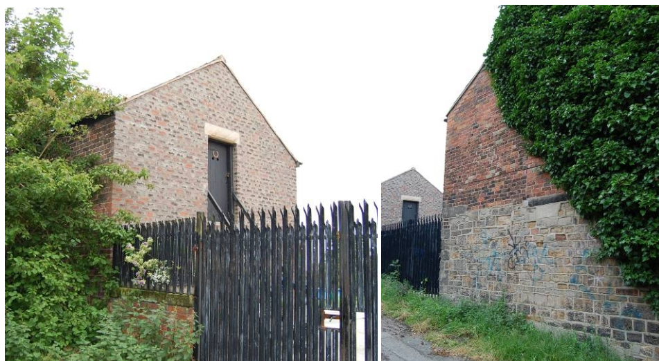
(left and right) poor quality pointing to stone and brickwork as well as highly detrimental palisade fencing at Ivy Farm.
